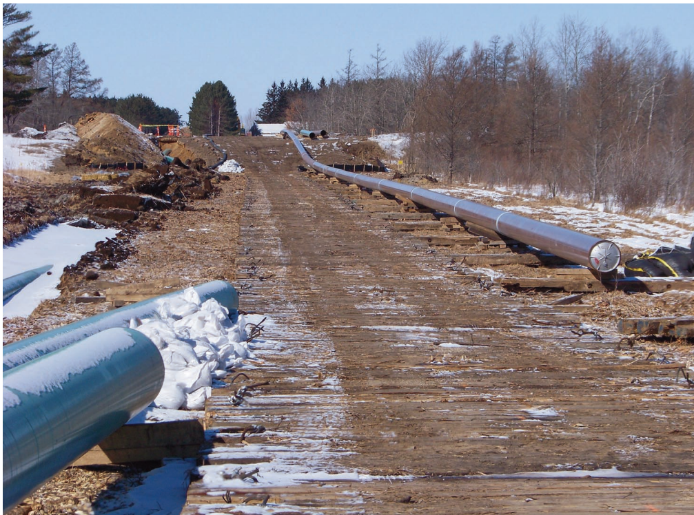
Figure 2. Construction mats helped protect the environment and heavy equipment traverse wet and thawing conditions along the ROW.
